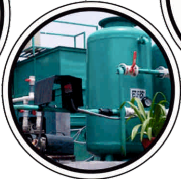
STP & ETP (CONSULTANT & MANUFACTURE)
